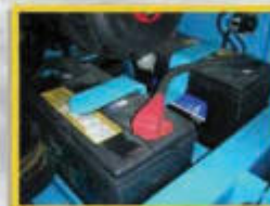
High power batteries for engine ignition.
